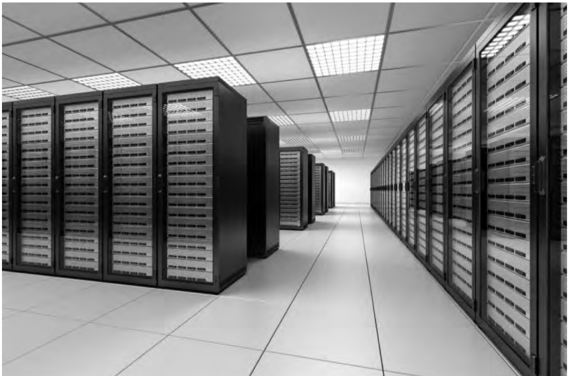
FIGURE 1.7 One server farm with more than 1000 servers
